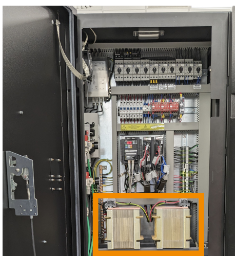
Figure 70 Two transformers in the rear left-hand electrical cupboard
